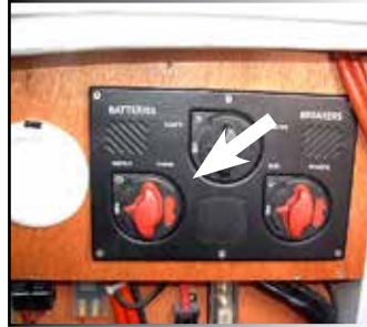
STARBOARD ENGINE CUT OUT
