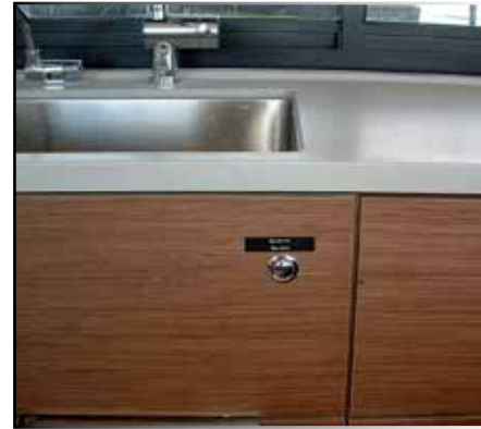
SEAWATER PUMP SWITCH
