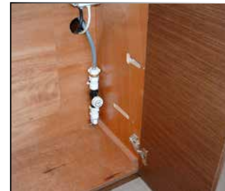
DISHWASHER FRESH WATER SUPPLY VALVE
