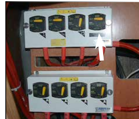
DAVIT AUTOMATIC BREAKER
