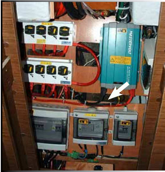
CONSUMING APPLIANCES CIRCUIT BREAKERS
